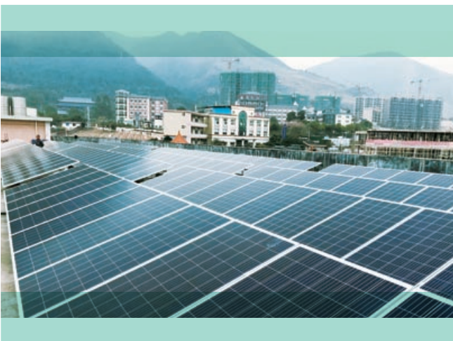
16 MW project in Liannan Yao Autonomous County
