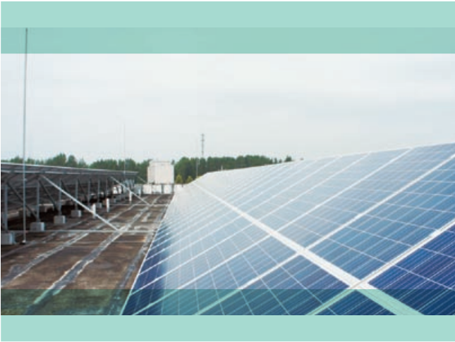
41 MW project in Ruyang County
